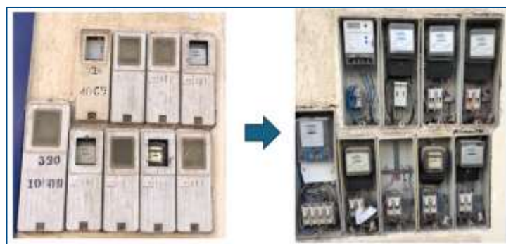
Figure 30- ONEE Exemple de coffret de raccordement BT
